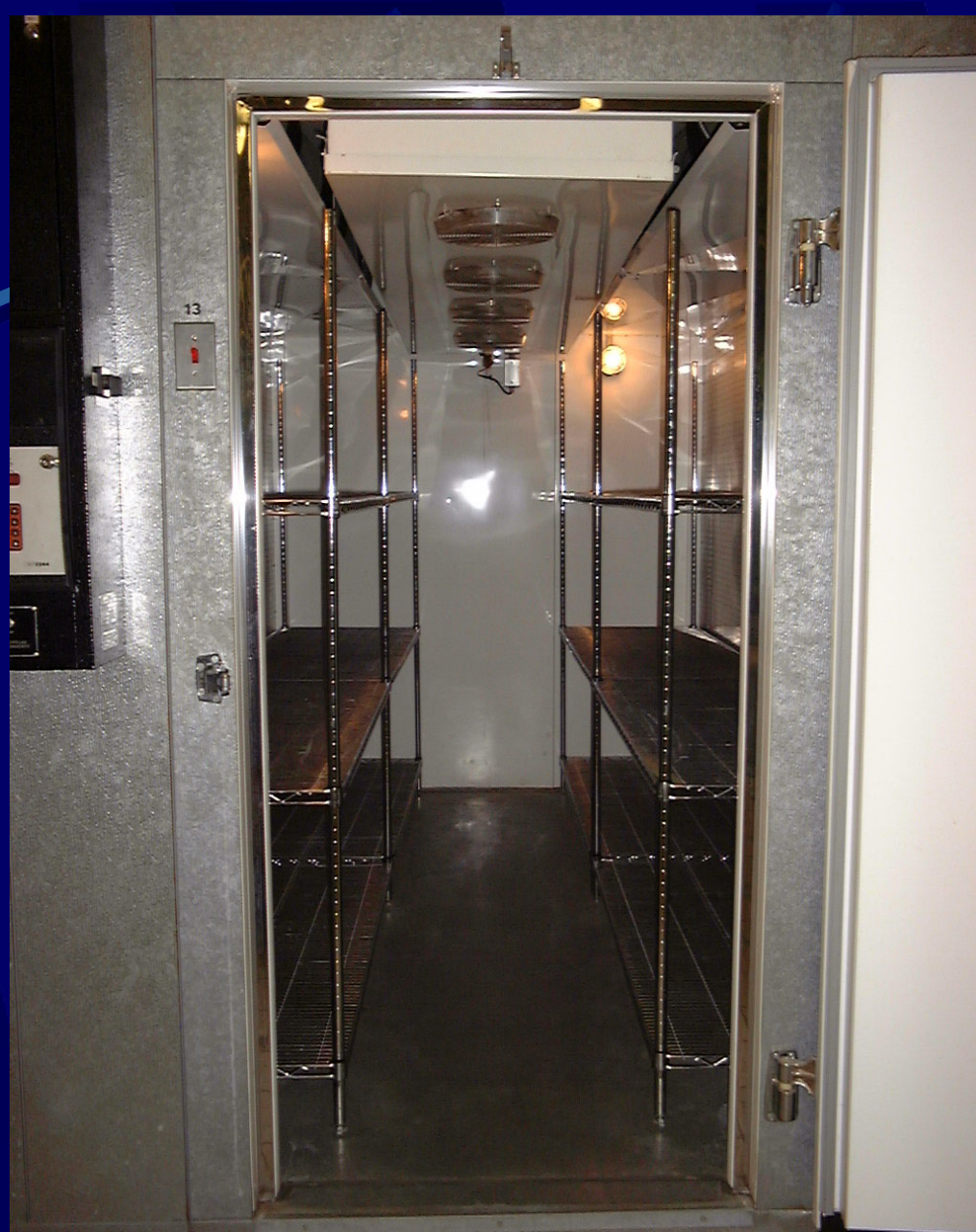
The C-812 cold room
